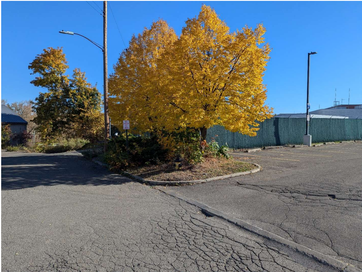
Figure 8: Overgrowth at Western End of Old Village Hall Lot and Surface Cracking (October 2024)
