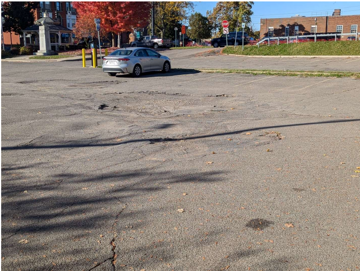
Figure 4: Isabelle Lot Cracking and Cratering (October 2024)
